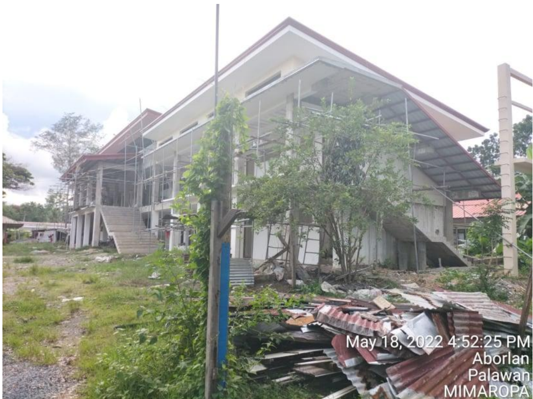
Rehabilitation and Furnishing of College of Community Development Building at Main Campus
